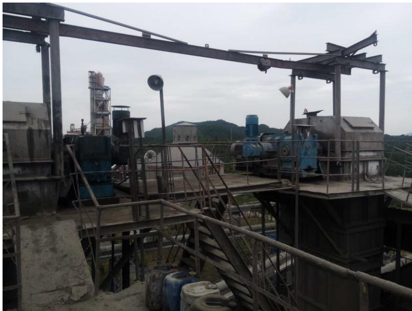
Reducers in cement plant
